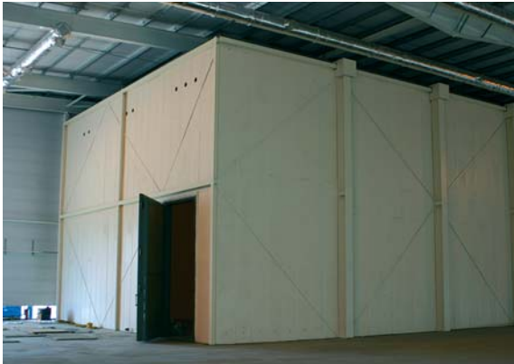
The front and side of the fully assembled strongroom, with the strongroom door at the front
